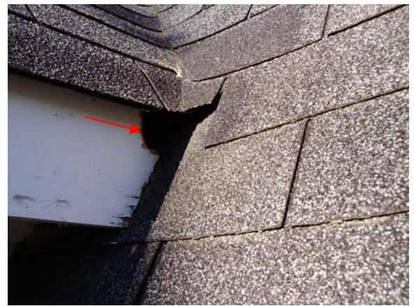
A rodent access hole has been chewed in the rear portion of the fascia board on the right side of the right dormer on the front of the home.
