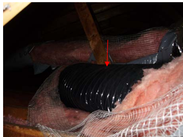
The insulation is damaged around several of the hvac supply ducts in the upper portion of the attic.
