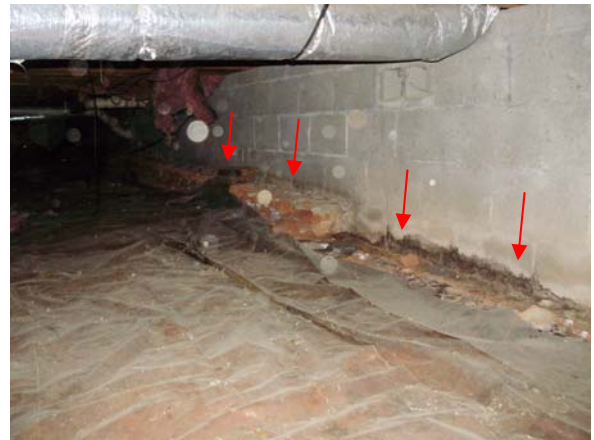
Past moisture stains were present on the lower portion of the rear foundation wall in the crawlspace.
