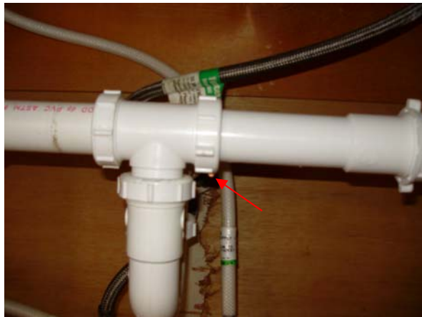
Repair the leak at the union in the plumbing drainpipe below the sinks in the master bathroom.
