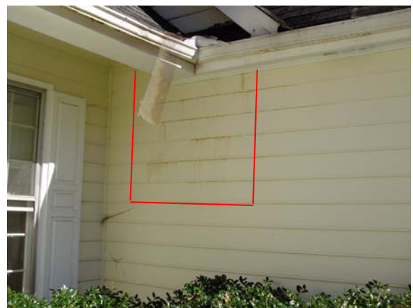
Several past moisture stains were present on the siding outside the left wall of the master bathroom.
