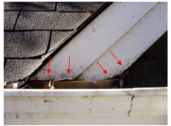
Moisture damage was noted at the fascia boards above the gutter at the bottom of the roof valley above the right wall of the master bedroom.
