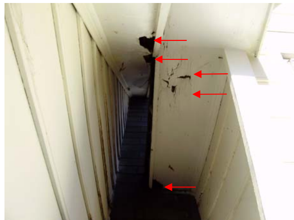
Rodent access holes and moisture damage was noted at the soffit boards on the left side of the left dormer on the front of the home.
