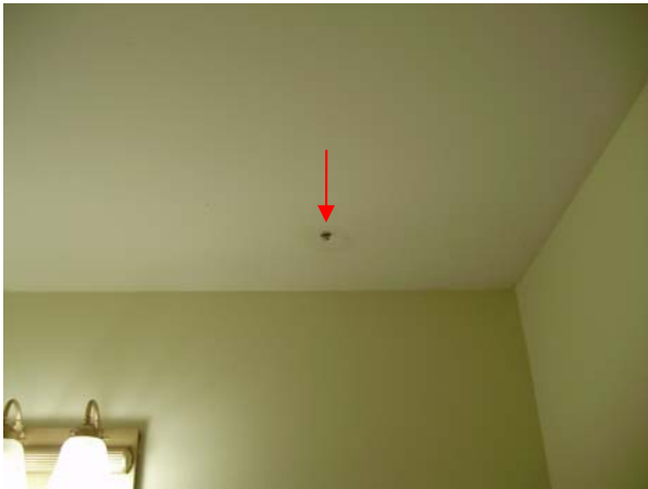
Moisture damage was noted at the sheetrock ceiling above the commode in the half bath, due to an active leak at the commode in the upstairs hall bathroom.
