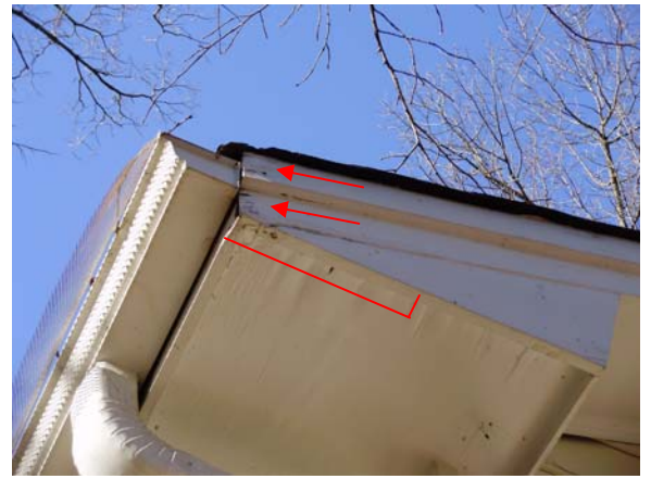
Moisture damage was noted at the fascia/soffit boards behind the gutter at the right corner of the front porch.
