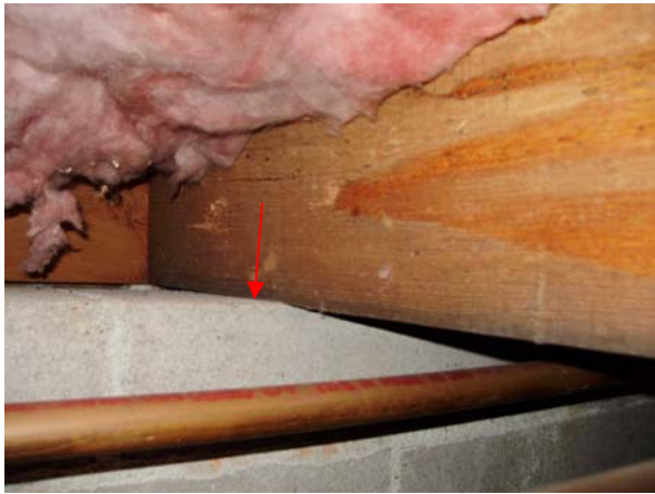
Pressure-treated sill plates were not installed above the foundation walls in the crawlspace.
