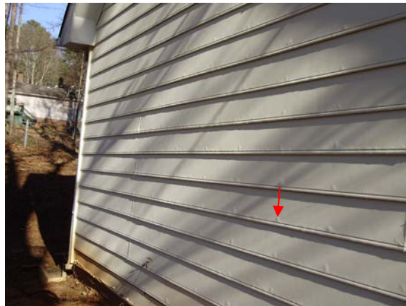
Swelling was present around the nail heads and along the lower edge of various pieces of siding on the left side of the garage.
