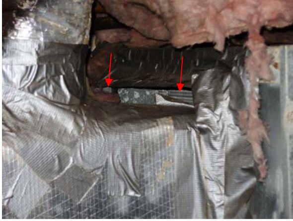
The supply plenum on the left side of the main floor furnace is loose (visible in the crawlspace).
